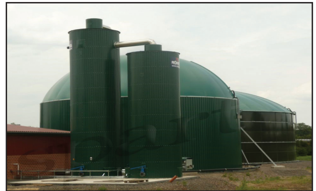
Example of an anaerobic digester that processes food scraps and other organic materials deemed acceptable by the operator.
